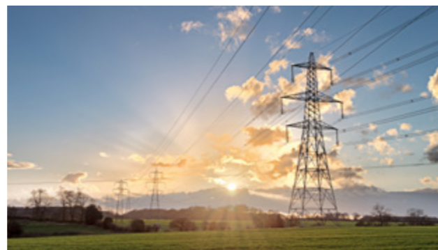
Ilm Electricity Transmission Line Canada
